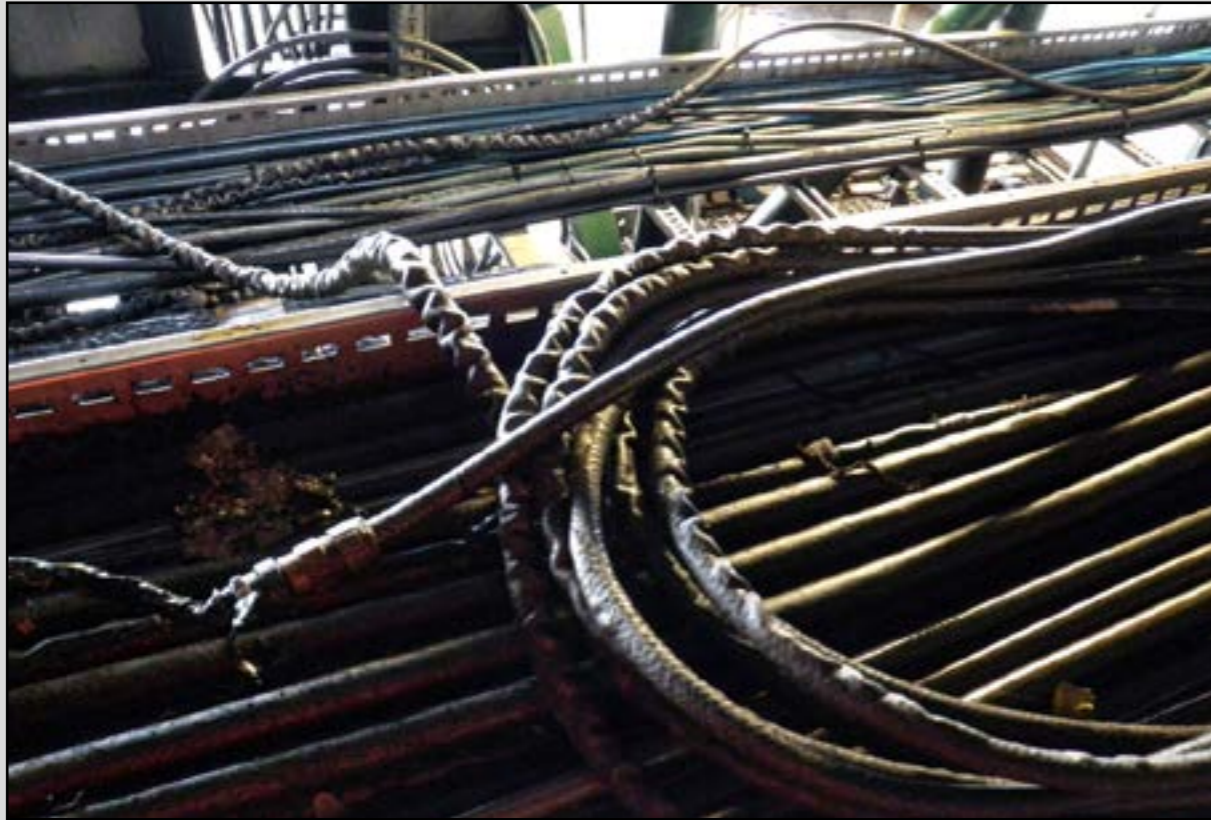
C2 Damaged sheath softened or even wrinkled sheath due to contaminates
