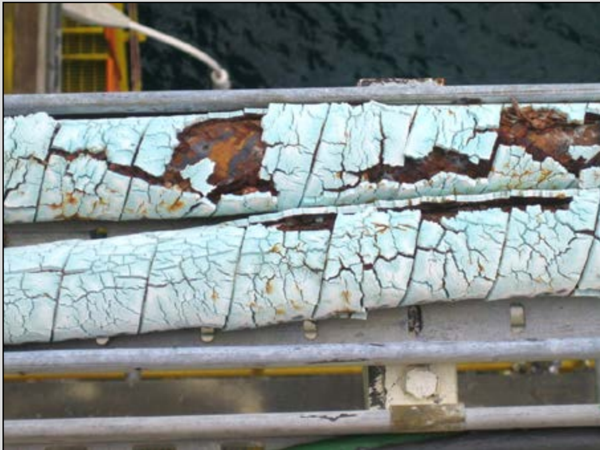
UV6 Cracked sheath, rusting armour
