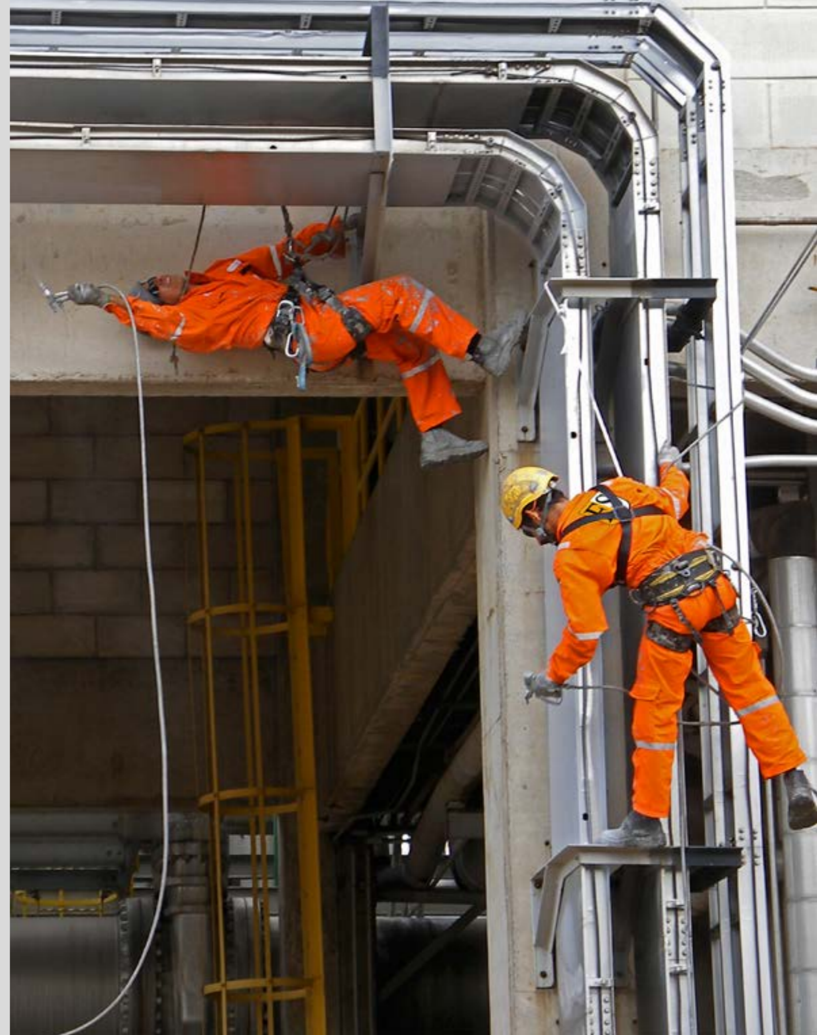
Fire Security's coating applicators employing rope access techniques to ensure total coverage for our clients turnkey cable maintenance operations.
